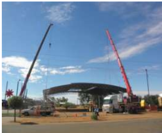
The roof of the new covered sports facility being lifted into place, April 2013
