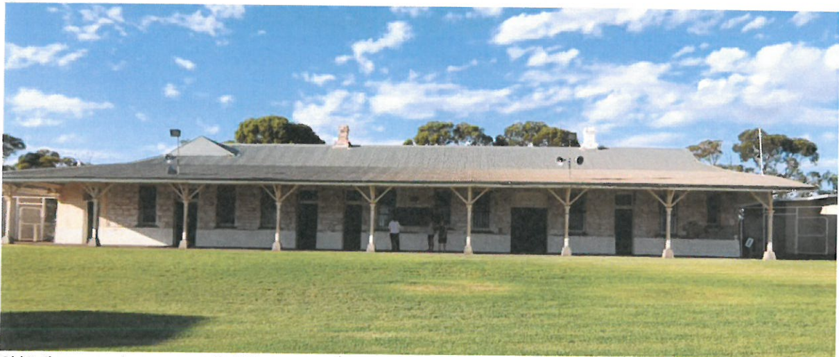
Old Railway complex now part the Yalgoo Racecourse: Bad restoration and rising damp problems
