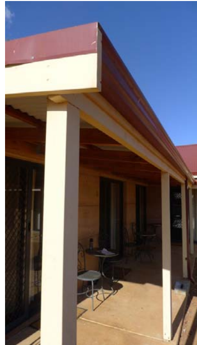
Eaves detail showing verandah beam shadowline accent strip gutter barge and capping, posts
