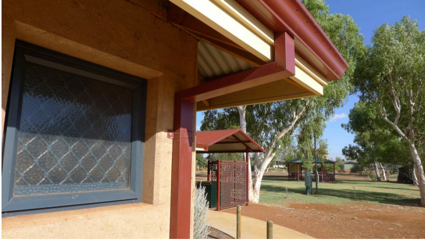
Detail showing 19mm chamfer around openings in rammed earth, gutters and fascia detail including shadow line accent strip, security screen, window frame colour and style.
