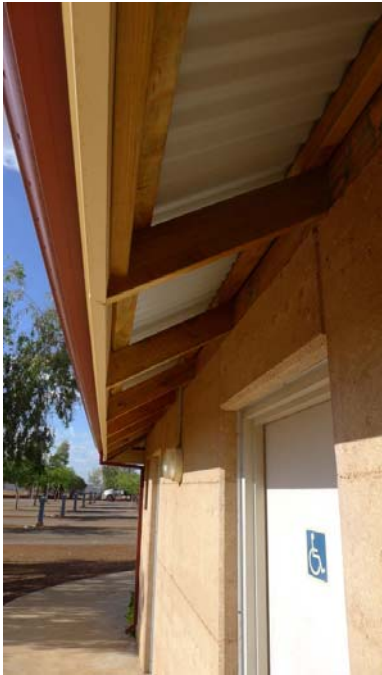
Eaves detail showing exposed unpainted eaves rafter tails and bird boards. Fascia and Gutter colour.
